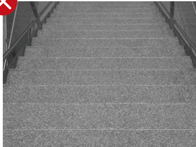
Poor Visual Contrast No Stair Nosings – Don't Take the Risk
