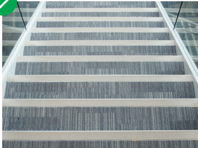
Good Visual Contrast Installed with Gradus Stair Nosings
